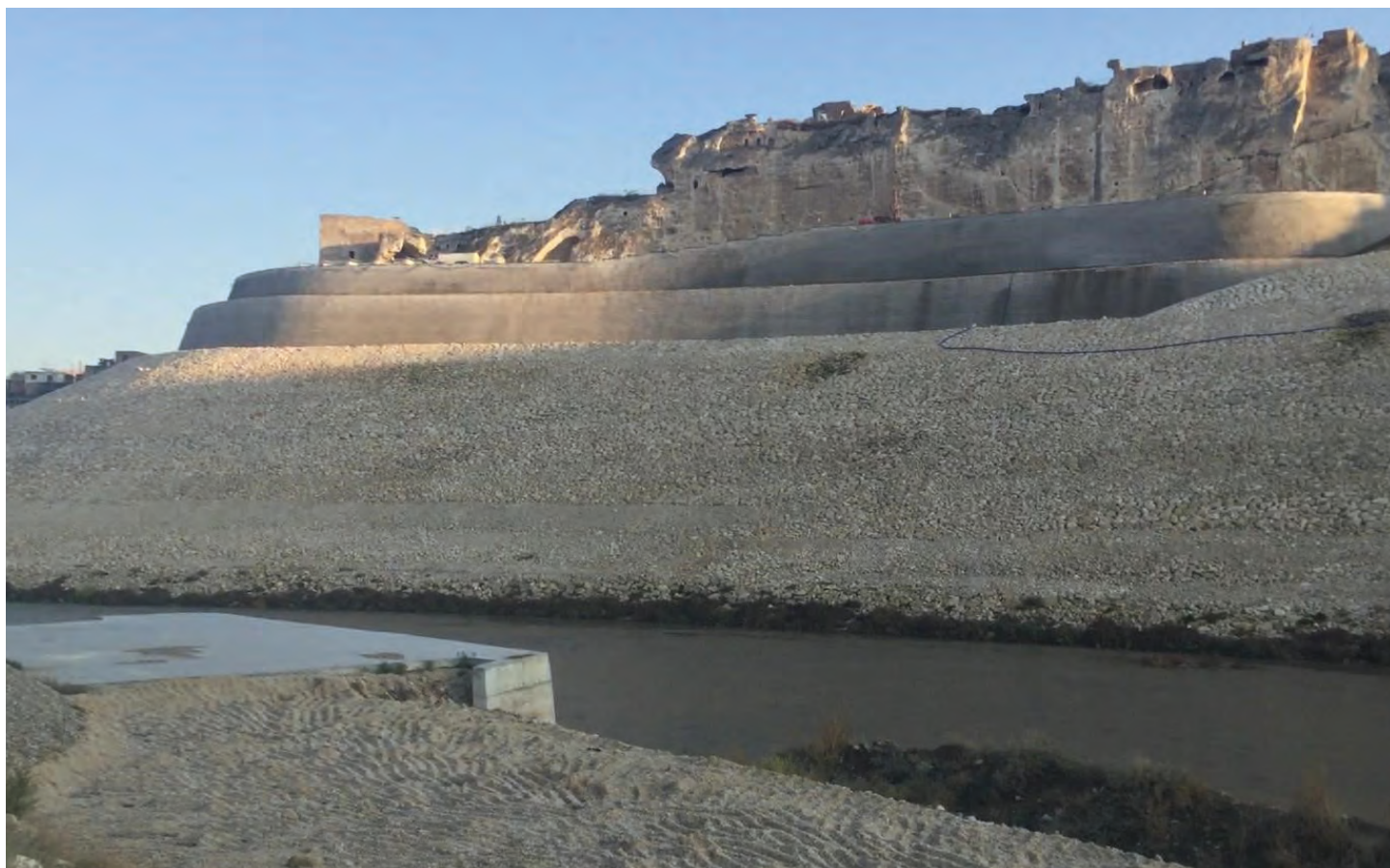
Last day of demolition of Hasankeyf settlement due to the İlisu dam construction, 03.11.2019 (photo by Pelin Tan)
